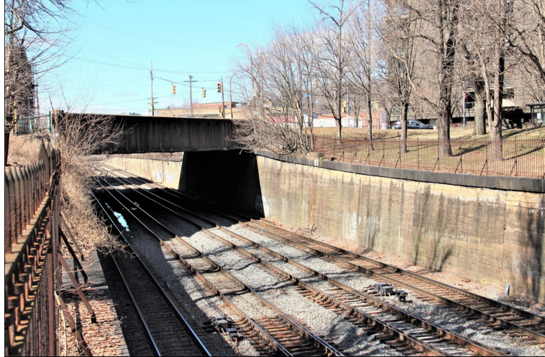
Photo of existing W. North Avenue Bridge from track edge, facing northwest.
