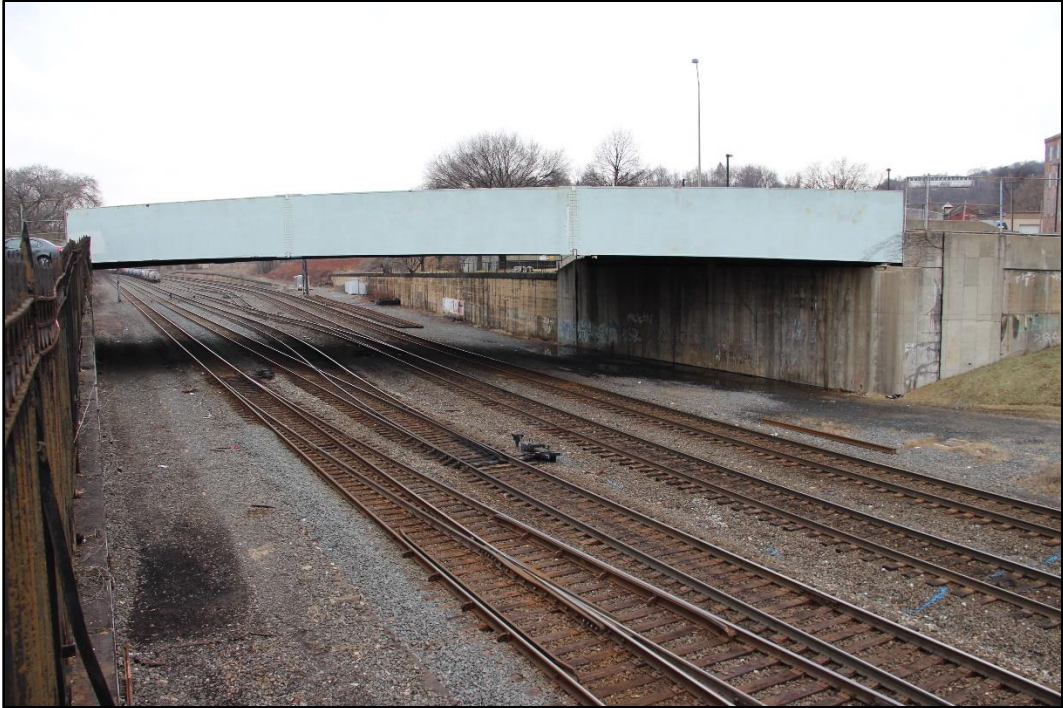
Figure 6-3: View of surveyed segment of rail corridor from northern terminus of Galveston Avenue showing the southeast side of the Pennsylvania Avenue Bridge and the northeast concrete and stone retaining walls (beyond the bridge), facing northwest.
