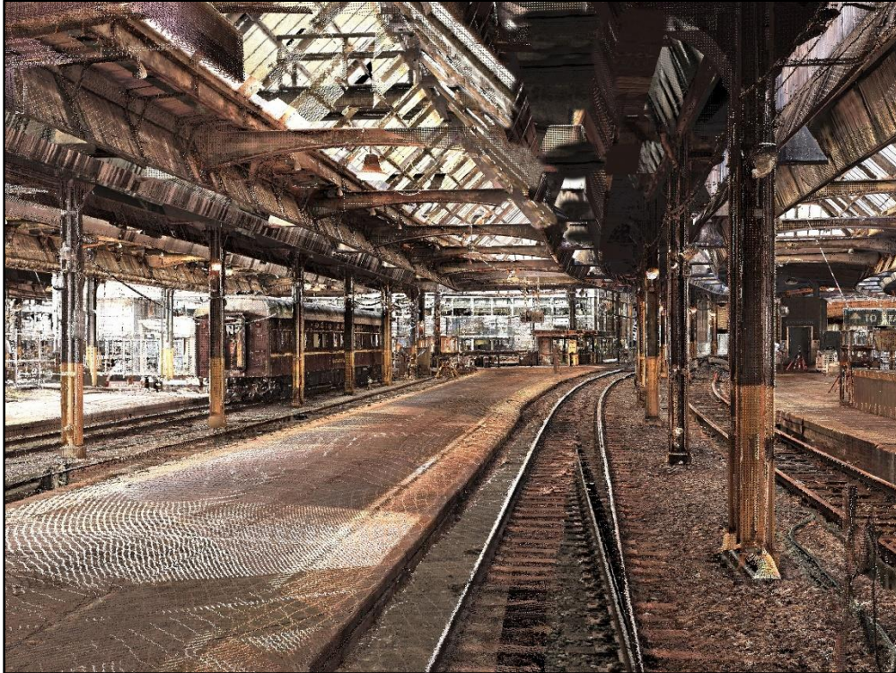
Figure 4-19: Photo of existing girders and exhaust chutes over Track 1 through trainshed, facing southwest.
