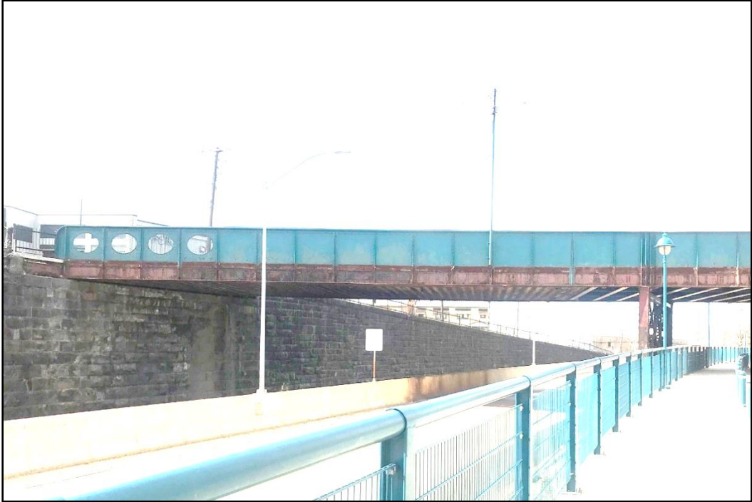
Figure 3-2: Washington Avenue Bridge showing southeast profile, southwest stone abutment, and steel center bent, facing northwest
