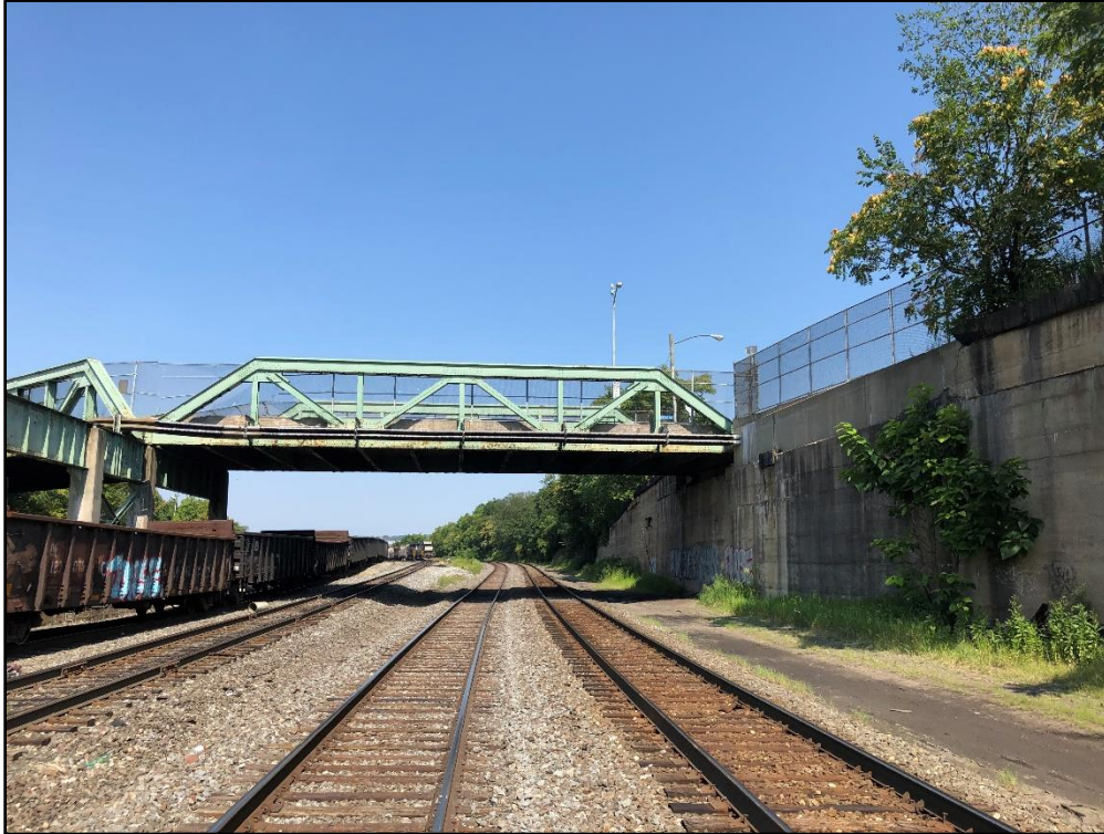
Figure 7-12: Photo of existing eastern-most main line tracks under the Columbus Avenue Bridge, facing northwest.
