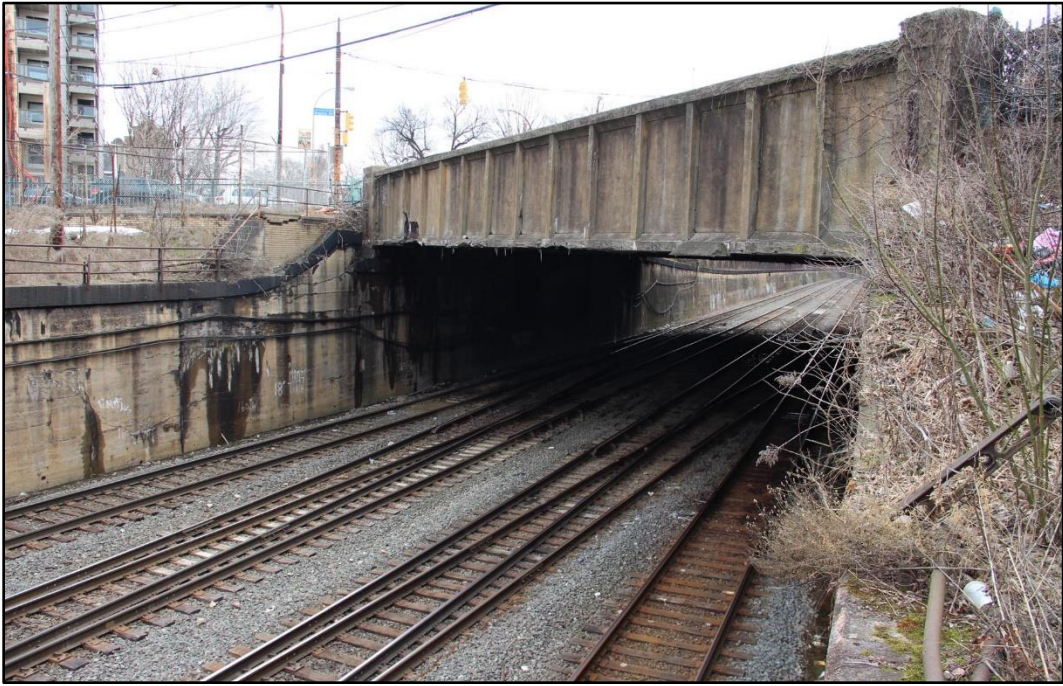
Figure 5-5: Detail of northwest girder of the 1929 W. North Avenue Bridge and view of the northeast concrete and stone retaining wall and standard railroad safety fencing, facing east.
