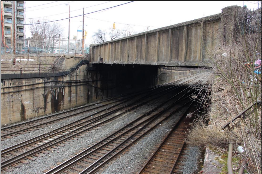
Figure 5-37: Photo of existing W. North Avenue Bridge from track edge, facing east.
