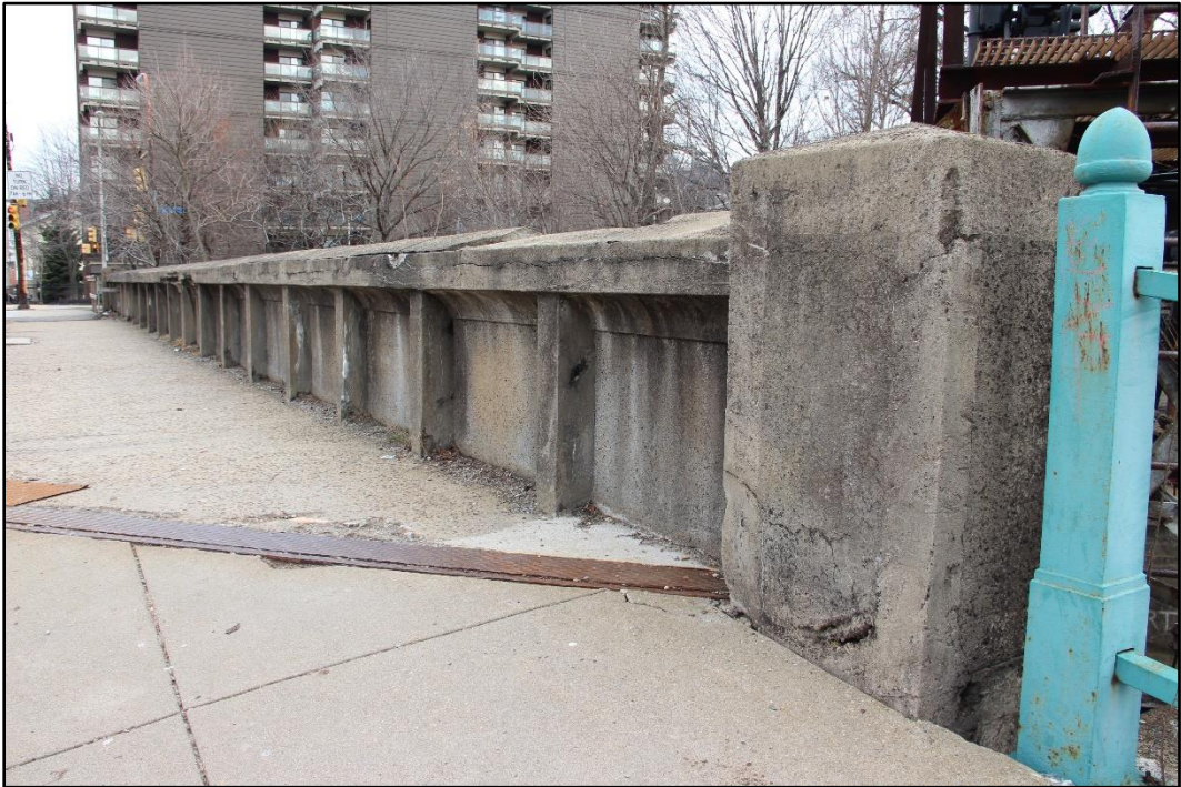
Figure 5-7: Detail of southeast girder of W. North Avenue Bridge from deck showing gunite finish and concrete end posts, facing north.
