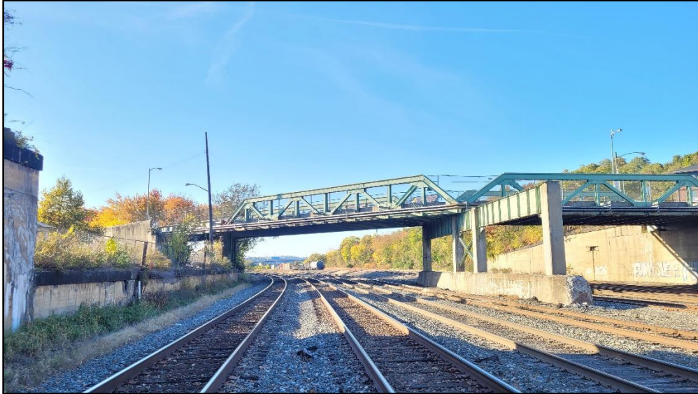
Figure 7-16: Photo of existing western-most main line tracks under the Columbus Avenue Bridge, facing northwest.
