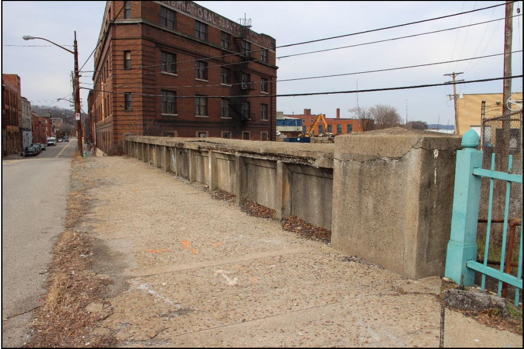
Figure 5-6: Detail of northwest girder of W. North Avenue Bridge from deck showing gunite finish and concrete end posts, facing west.
