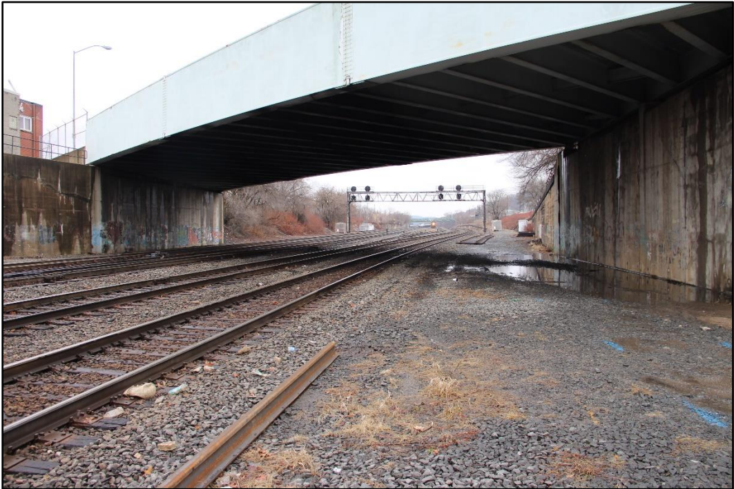
Figure 6-8: Southeast side of the Pennsylvania Avenue Bridge showing the modern substructure and superstructure, facing northwest.
