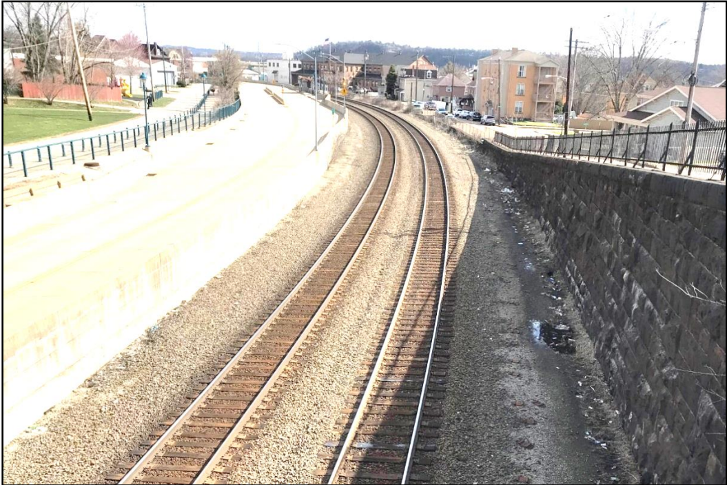
Figure 3-5: Detail of stone retaining wall and wrought-iron fencing of the Palmer Street south approach ramp, facing southeast.
