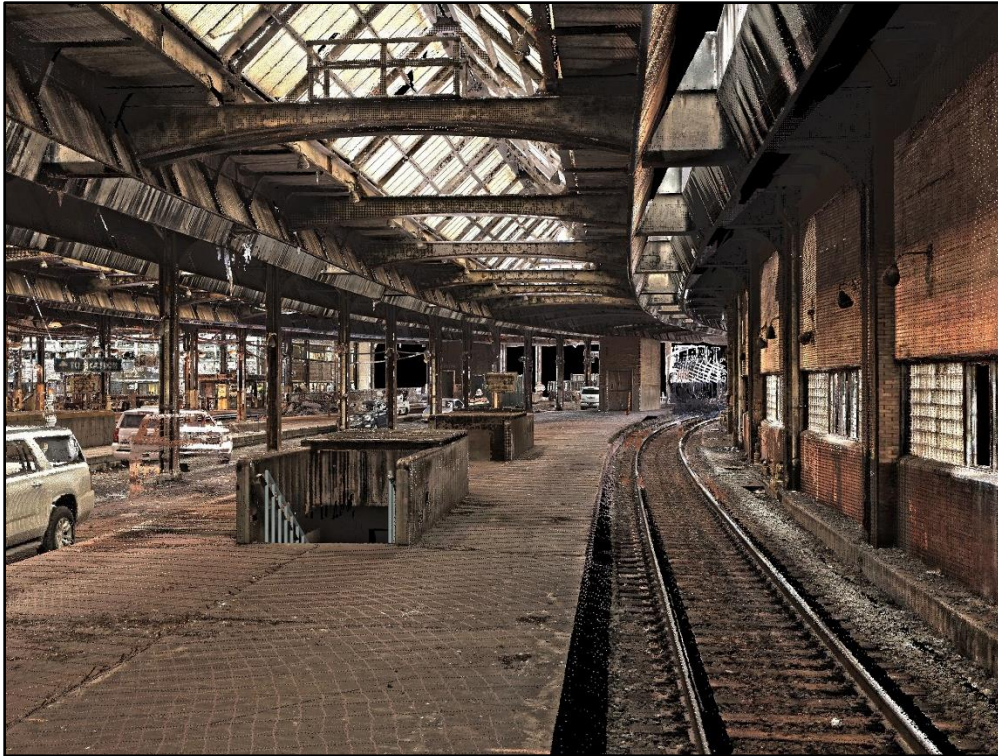
Figure 4-21: Photo of existing girders and exhaust chutes over Track 2 through trainshed, facing west.
