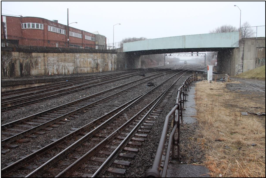
Figure 6-2: View of surveyed segment of rail corridor from western terminus of Riversea Road showing the southeast side of the Pennsylvania Avenue Bridge, the southwest concrete retaining walls with stone coping (left), decorative wrought iron fencing (left), and standard railroad safety fencing (center-right), facing northwest. Ramps for former elevated sidings are visible on both sides of the corridor.
