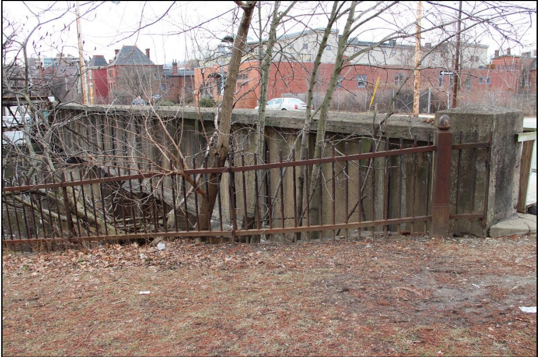
Figure 5-4: Detail of southeast girder of the 1929 W. North Avenue Bridge with a segment of 1929 iron fencing along the northeast side of the corridor, facing southwest.
