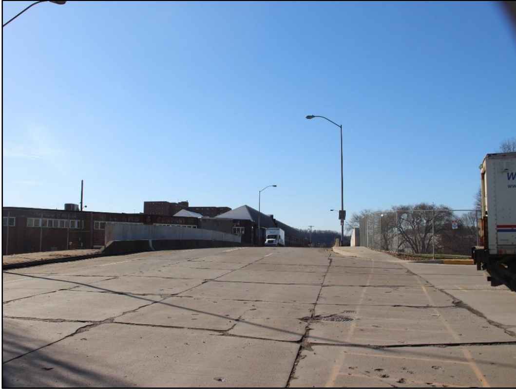
Figure 6-21: Photo of existing Pennsylvania Avenue Bridge from street level, showing 901 Pennsylvania Avenue in background, facing southwest.
