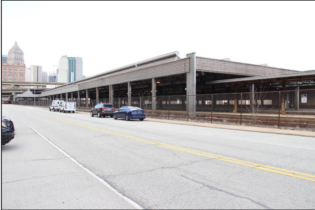
Figure 4-6: Northeast and southeast façades of contributing trainshed's northeast pavilion. At far right, an umbrella shed covers platform 3. View from Martin Luther King, Jr. East Busway, facing west.
