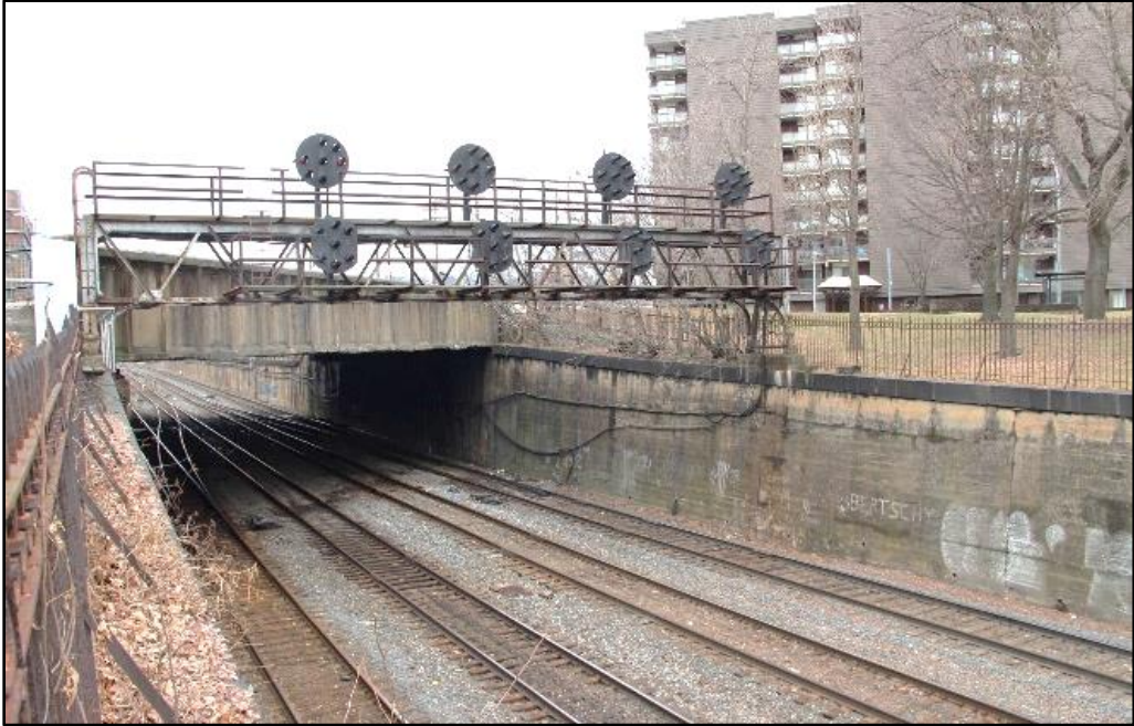
Figure 5-8: Railroad signal bridge (now removed) spanning depressed railroad corridor through Allegheny Commons Park, facing northwest.
