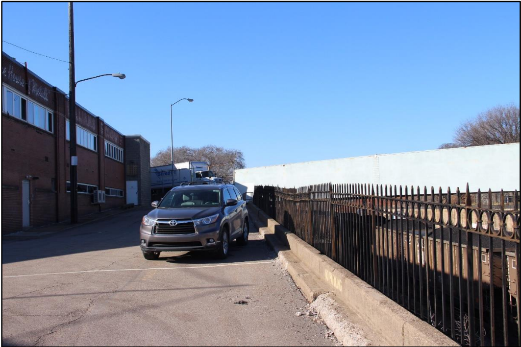
Figure 6-6: Detail of wrought-iron fencing atop the southwest concrete and stone retaining wall along northeast side of Galveston Avenue, facing northwest.
