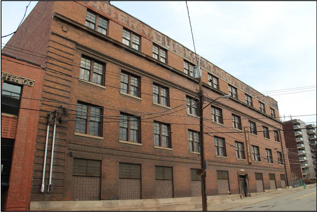
Figure 4-30: Current view of the International Harvester Building showing the stepped limestone foundation/water table and first floor windowsills of the three easternmost first-floor display windows after alterations from street grade changes ca. 1929 and again in the 1940s.
