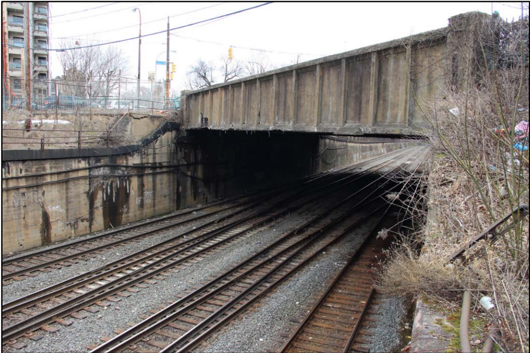
Figure 4-17: Photo of existing W. North Avenue Bridge from track edge, facing east.
