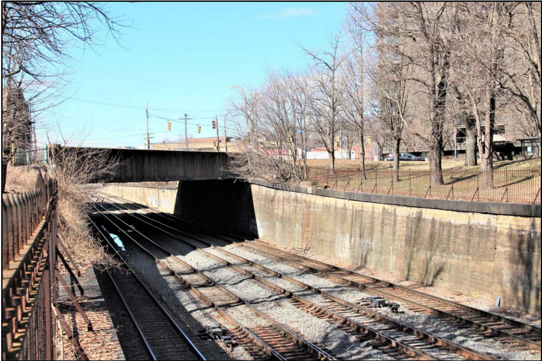
Figure 4-15: Photo of existing W. North Avenue Bridge from track edge, facing northwest.
